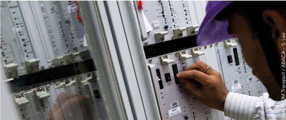
Railway - Closed from electrical operating areas
